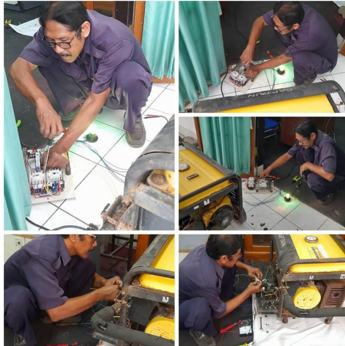
Gambar 2: Uji coba Panel ATS/AMF
